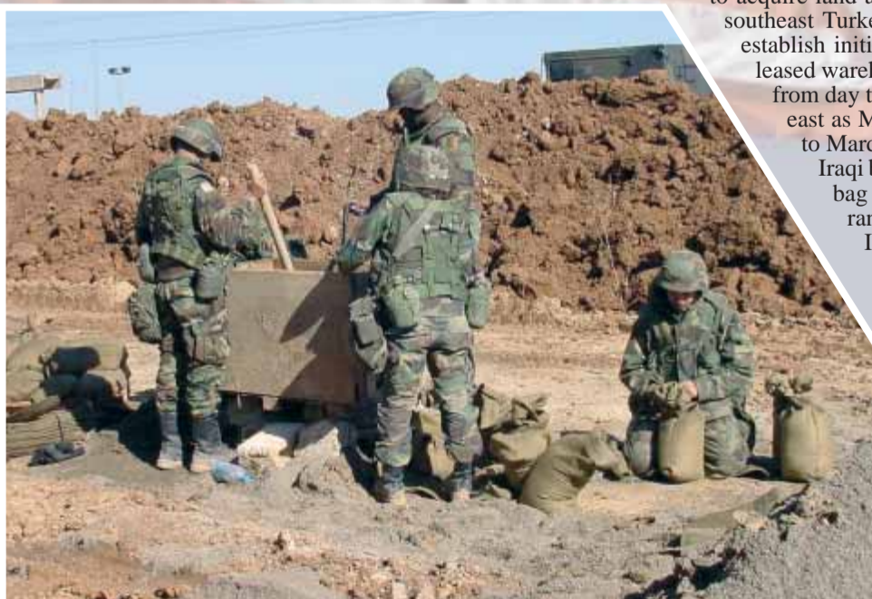
Soldiers from the 1st Infantry Division make force protection improvements at the ARFOR-T Headquarters in Mardin, Turkey.
